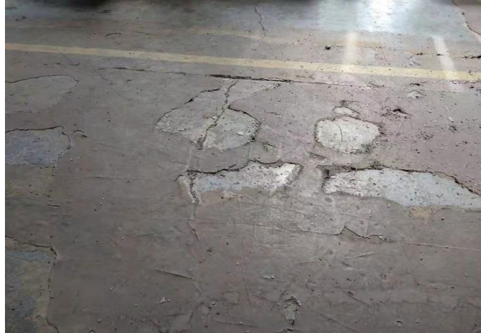
Figure 1 Secondary damage of concrete pavement after repair
